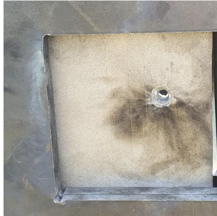
Fail: Full Penetration
