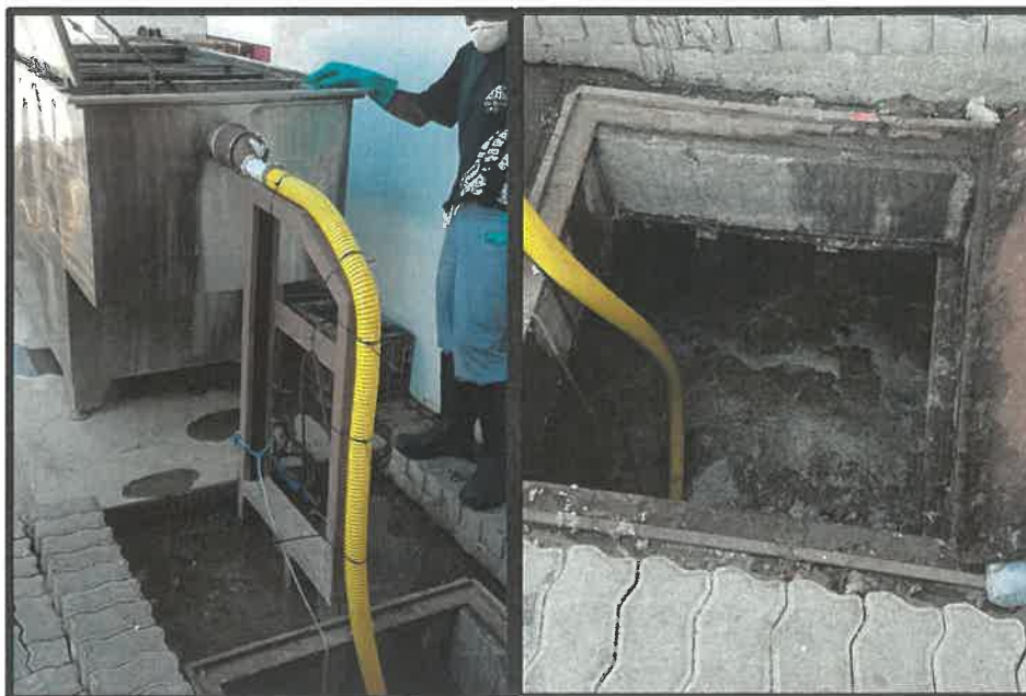
Figure 2.6: Effluent discharge point at the production site where the fat is mechanically separated from the water to prevent it from blocking the main municipal sewage line running from the plant to the wastewater treatment plant.
