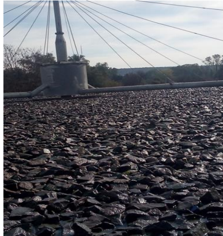
Figure 3.6 Trickling filter at the BWTW (Author's own, 2023)
