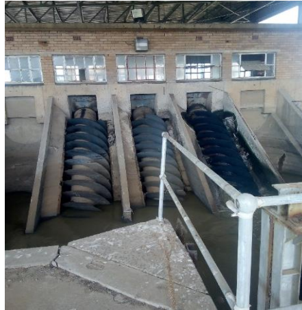
Figure 3.2 Screw pumps at the BWTW (Author's own, 2023)
