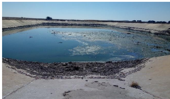
Figure 3.17 Sludge settling tank at the NEWTW (Author's own, 2023)
