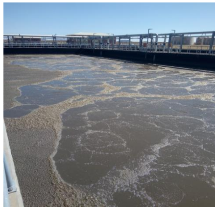
Figure 3.15 Aeration tank at the NEWTW (Author's own, 2023)
