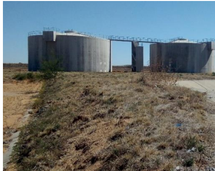
Figure 3.16 Digester tanks at the NEWTW (Author's own, 2023)
