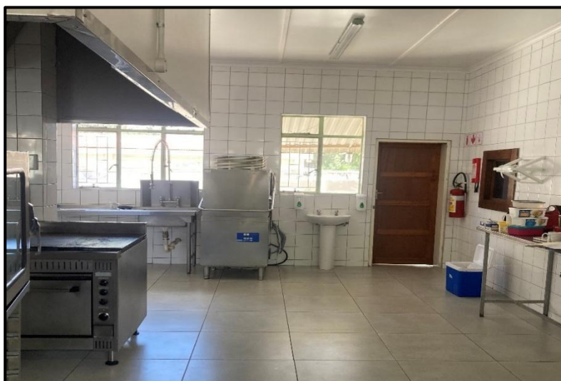
Figure 8: Handwash basin, stainless steel dishwashing area for utensils and cutlery, and a cooking stove located within the kitchen space, illustrating key components essential for maintaining hygiene and food safety compliance
