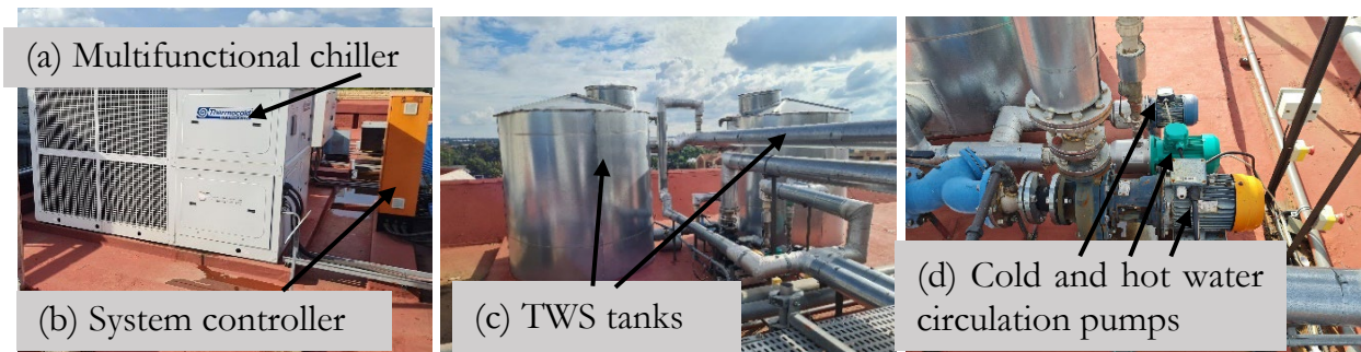
Figure 3.3. Heat recovery system installed at the Mediclinic Hospital, Bloemfontein.
