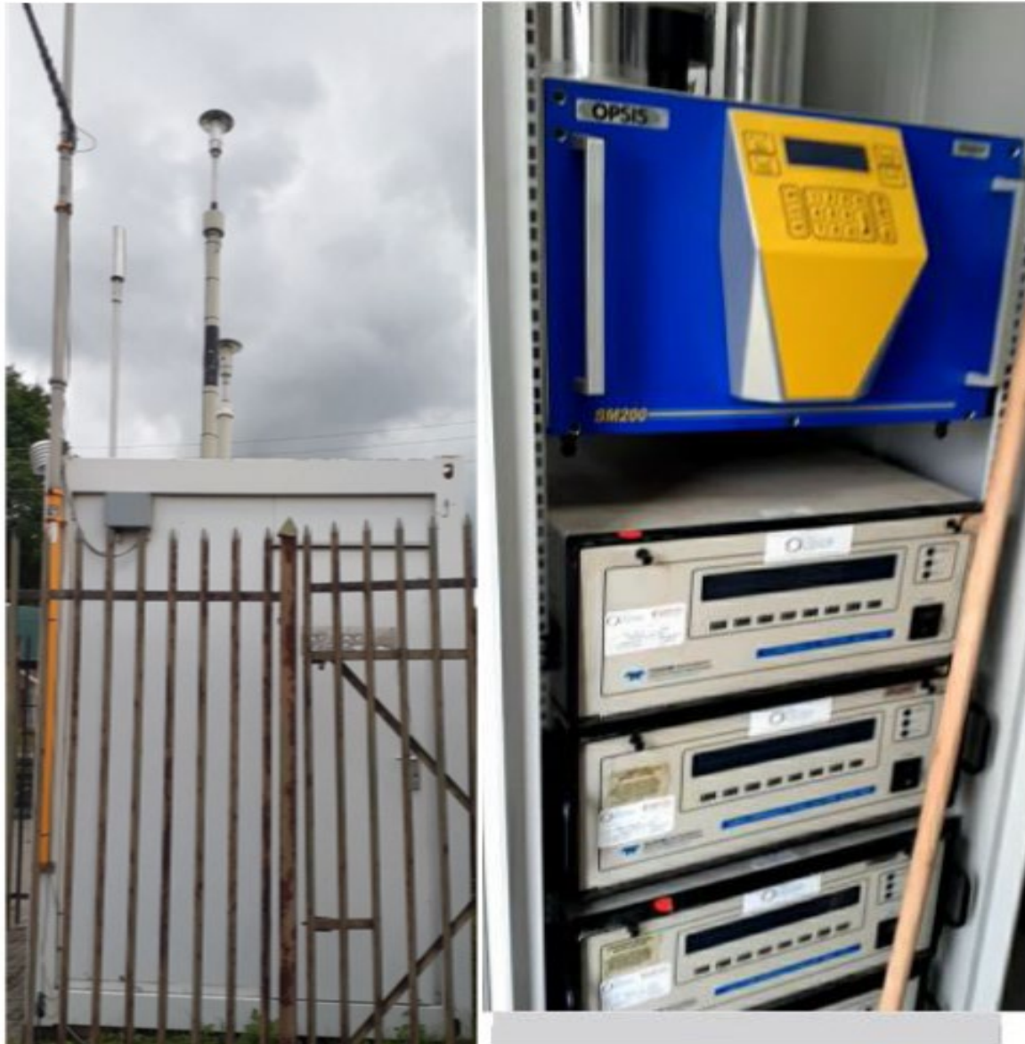
FIGURE 2.1: ON-SITE AIR QUALITY MONITORING STATION
