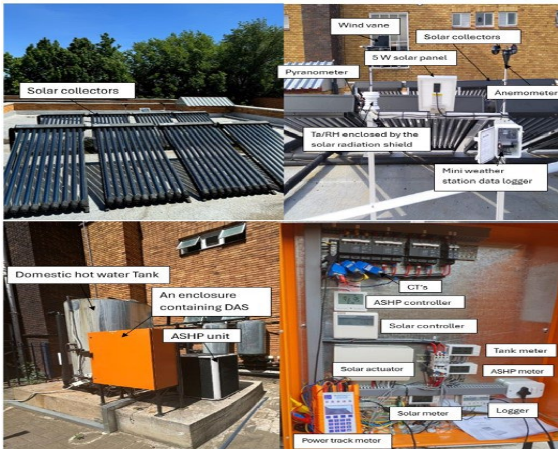
Figure 3:2: Designed and installed HSAASHP water heater
