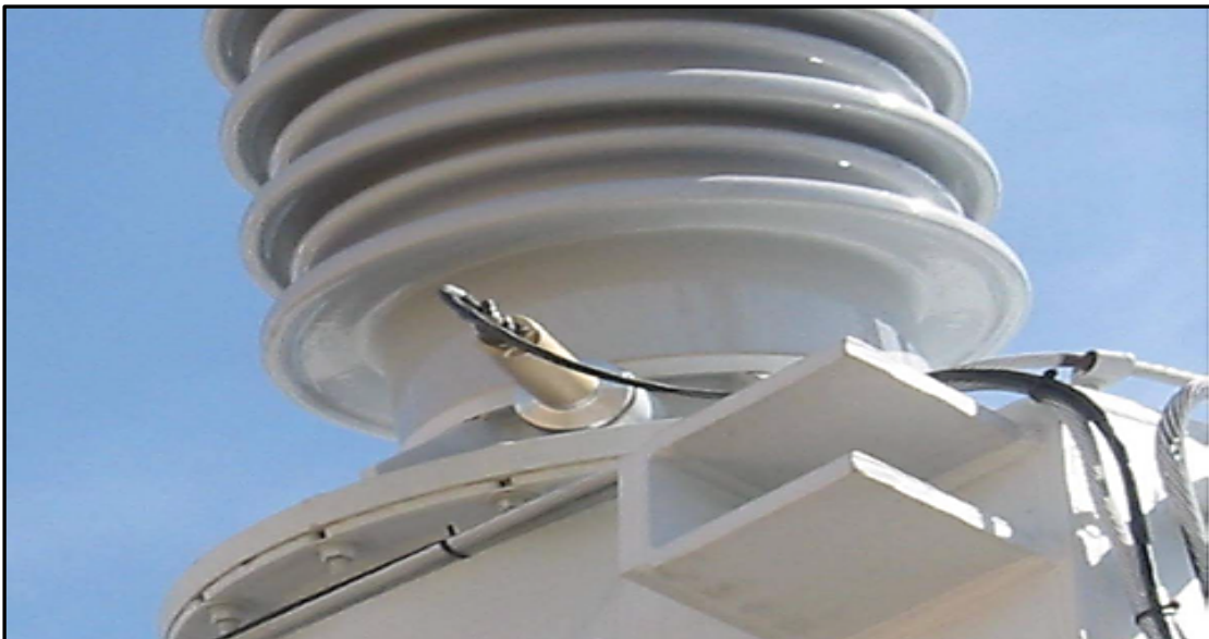
Figure 3.13 Sensor installed on an HV bushing test tap
