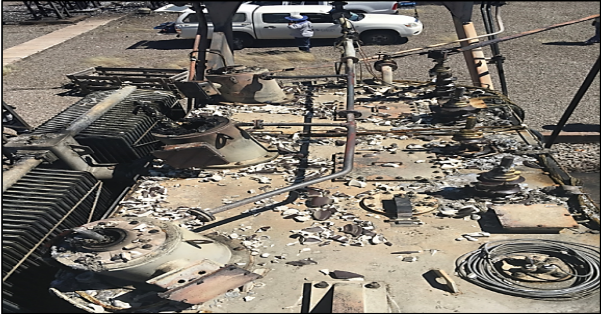
Figure 2.7: Failed exploded bushings resulted in a fire
