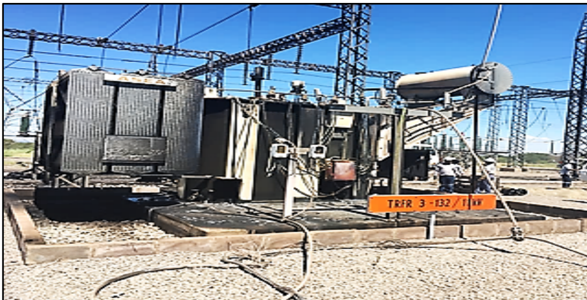
Figure 2.6: Failed exploded bushings resulted in a fire
