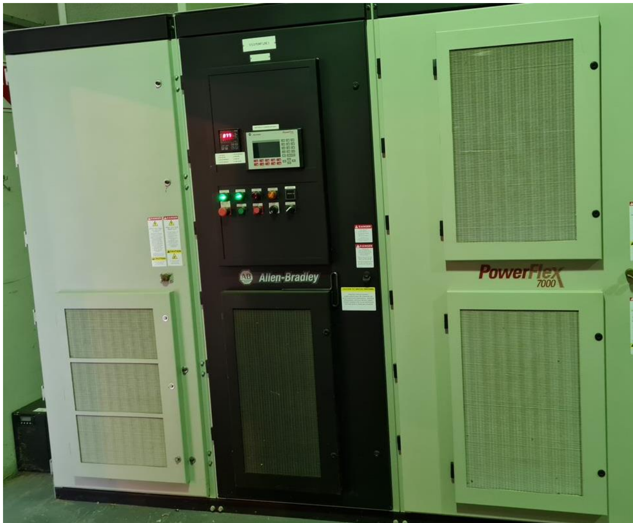
Figure B: Allen-Bradley VFD driver
