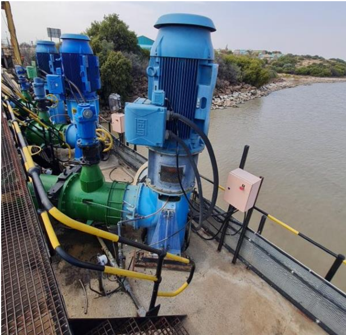
Figure 3.2: Electrical water pumps
