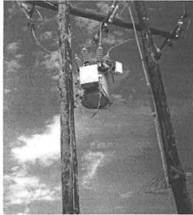
Fig. 6.1: A type KFE recloser, mounted on a pole structure, showing the external cabinet mounted on the side of the recloser.
