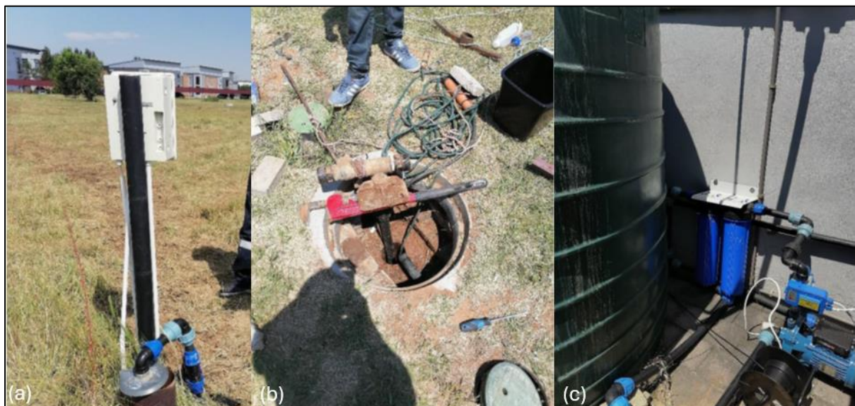
Figure 4.5 (a) Borehole 3; (b) Borehole 4; (c) Borehole 4 filter system seen at the inlet of the water into the 10 000 ℓ storage tank
