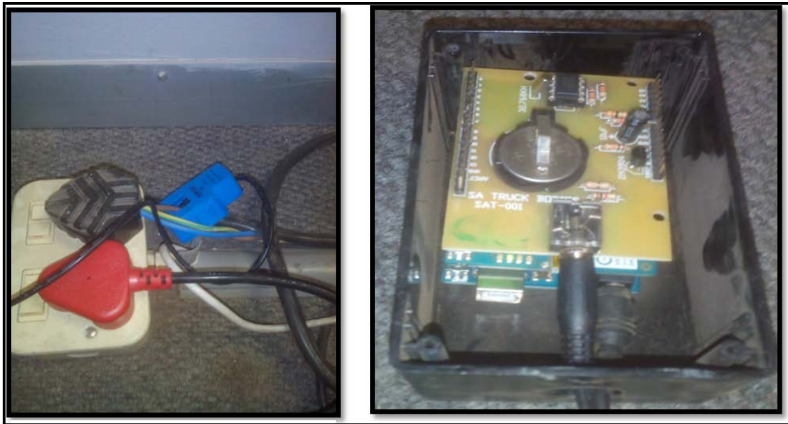
Figure 4-7: Node for real-time monitoring with CT on Live wire
