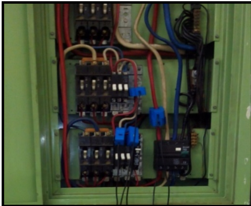
Figure 3-2: Current transformer on alternating current power lines
