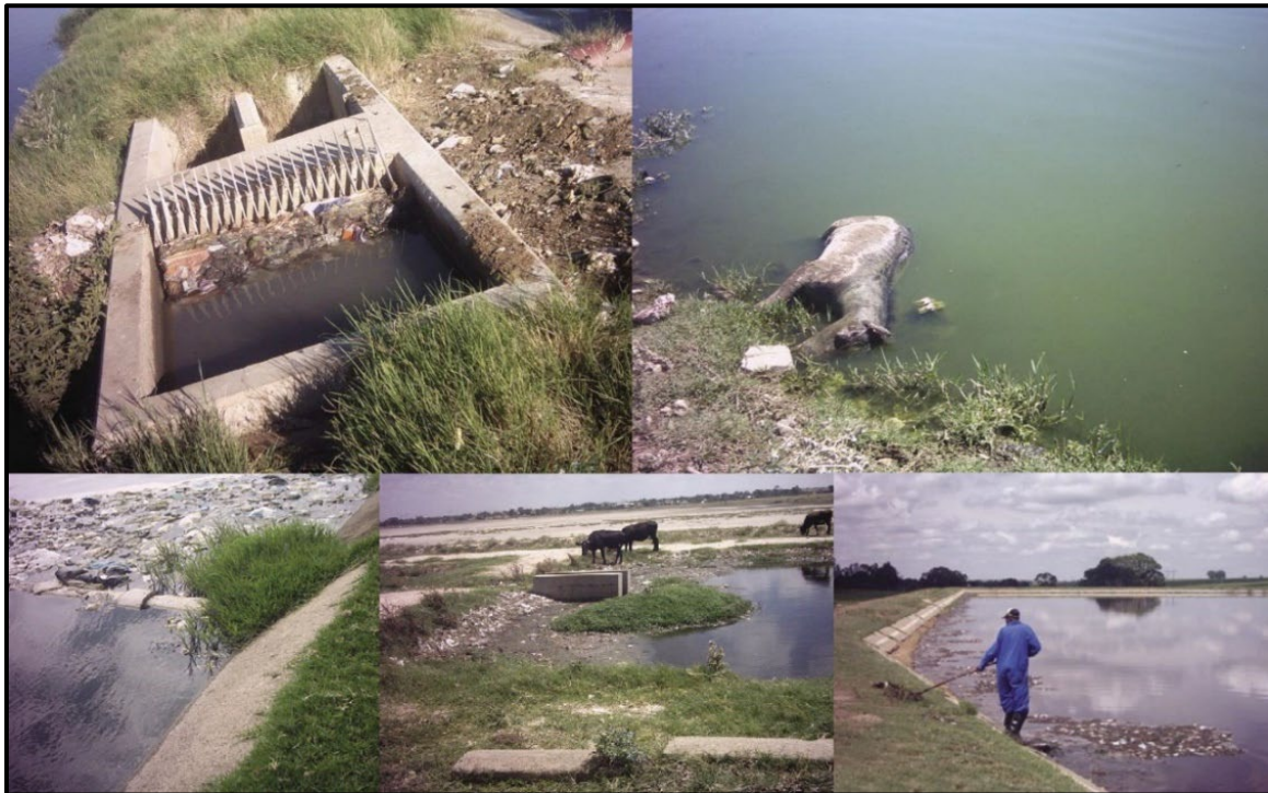
Figure 2.8: Dilapidated state of the WSP in the Nala (Bothaville) Municipality, FS province (Jack et al., 2006)
