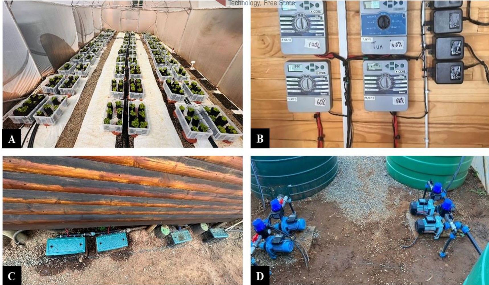
Figure 3.1: The irrigation setup (A) drip irrigation, (B) residential irrigation controller, (C) valves, and (D) tanks and pumps.
