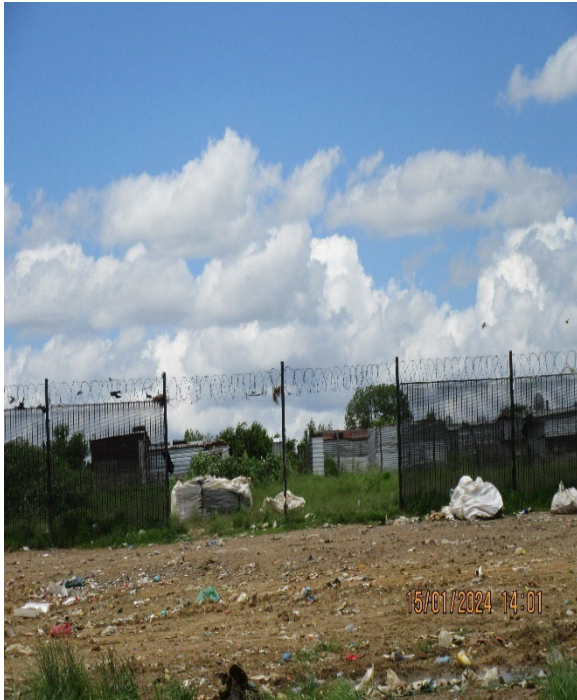
Annexure 1.7: Vandalised galvanised steel fencing with razor wire topping in the Harrismith landfill site
