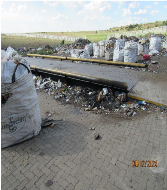
Annexure 1.20: A non-functional weighbridge in the Winburg landfill site
