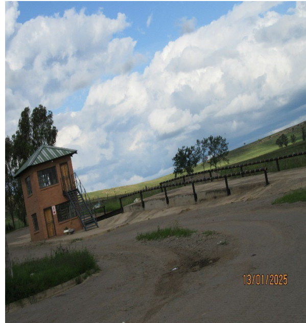
Annexure 1.21: A newly constructed but non-functional weighbridge in the Bethlehem landfill site
