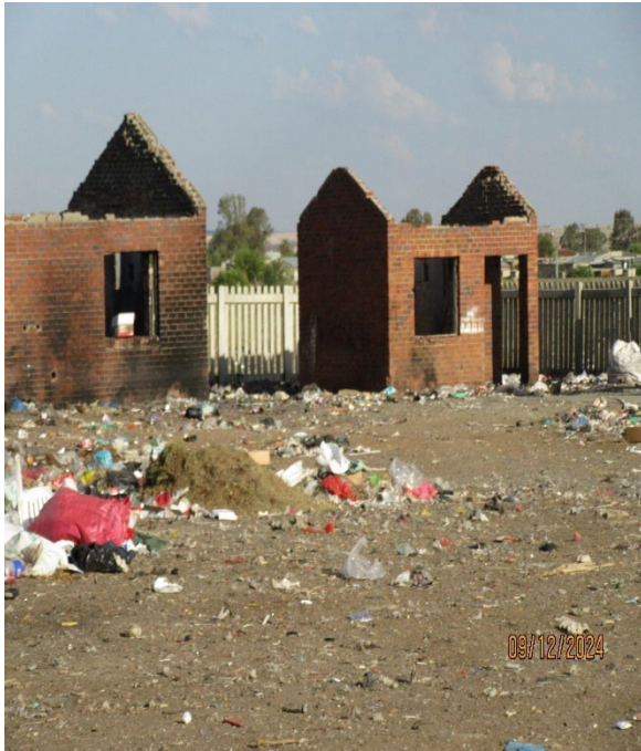
Annexure 1.11: The workers' office and ablution facility were burnt and vandalised at the Theunissen landfill site
