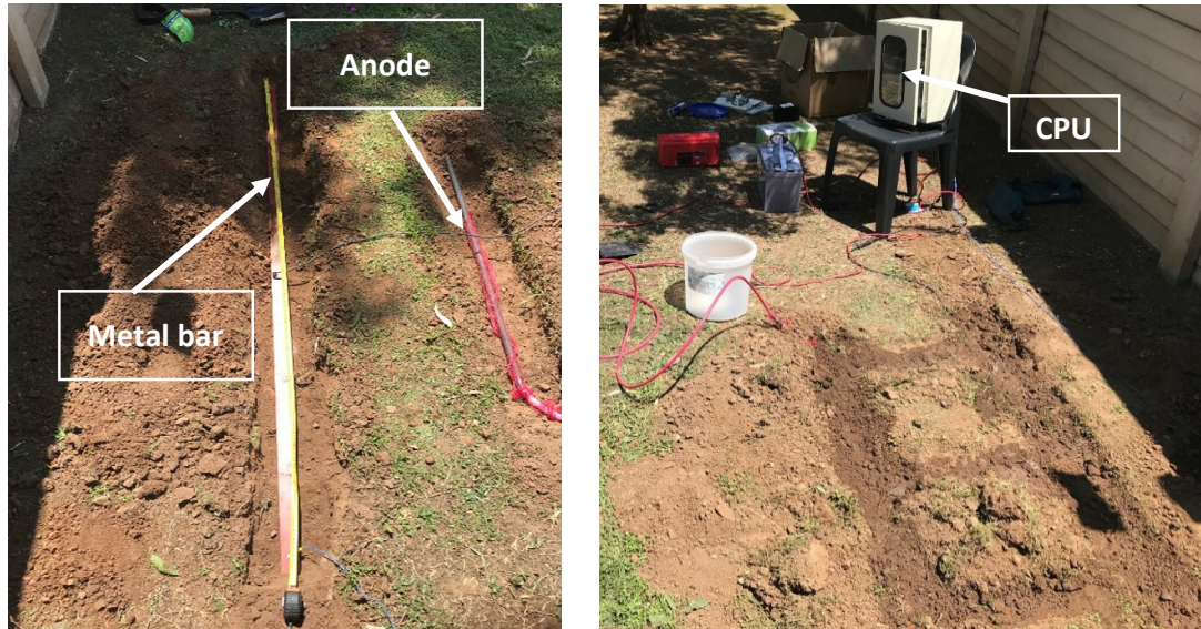
Figure 5.5: (a) left, ground installations, (b) right, Anode and metal bar installed.
