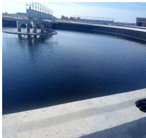
Figure 3.13 Secondary settling tank at the NEWTW (Author's own, 2023)
