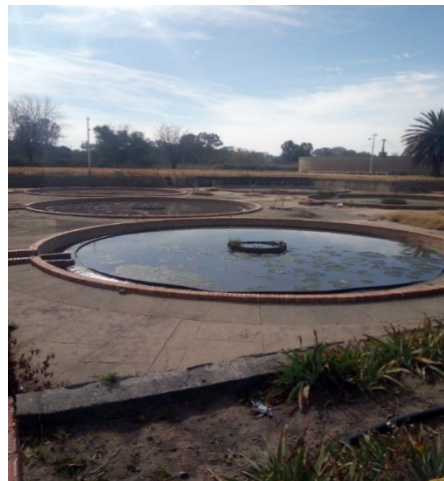
Figure 3.4 Primary settling tanks at the BWTW (Author's own, 2023)
