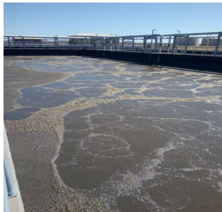
Figure 3.15 Aeration tank at the NEWTW (Author's own, 2023)
