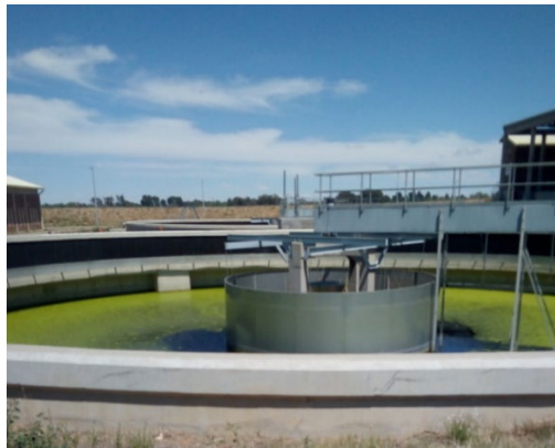
Figure 3.12 Primary settling tank at the NEWTW (Author's own, 2023)
