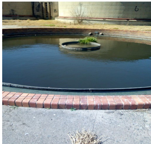
Figure 3.7 Secondary settling tanks at the BWTW (Author's own, 2023)
