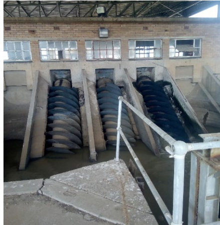
Figure 3.2 Screw pumps at the BWTW (Author's own, 2023)
