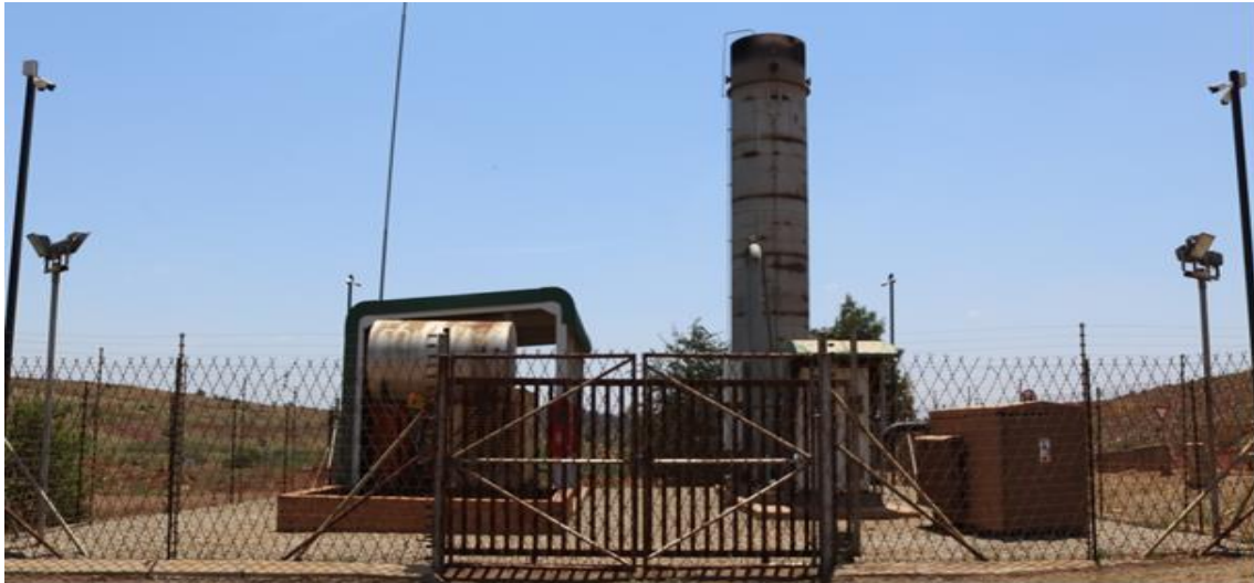
Figure 2.8: Energy generating plant at Gauteng waste disposal facility to manage gas
