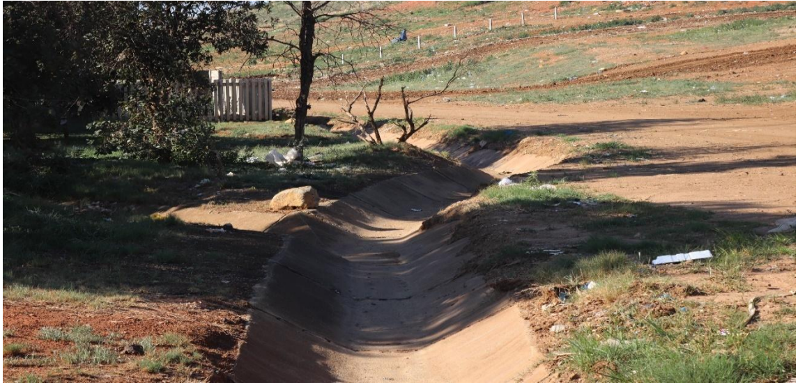
Figure 5.29: Channel to control stormwater at a landfill site in Gauteng province Source: Noe, 2018
