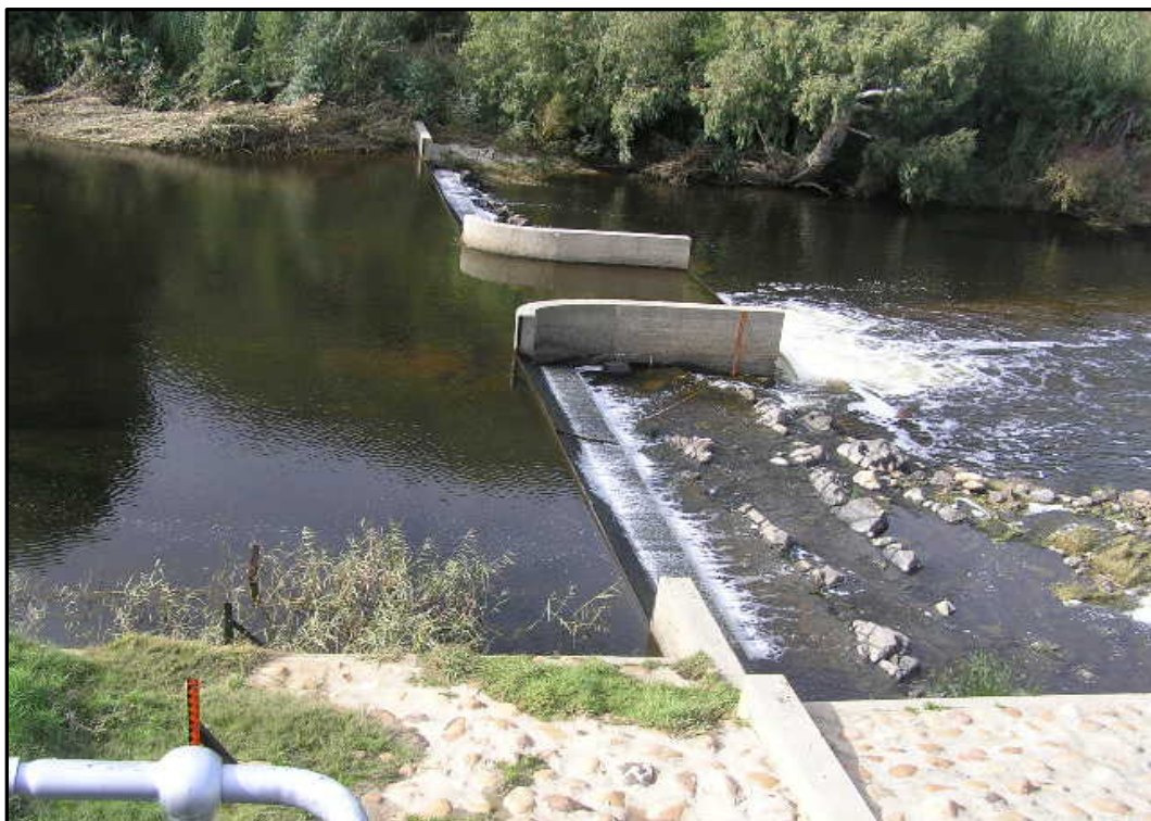
Figure 5.13: Gauging weir H5H004 in the Breë River
