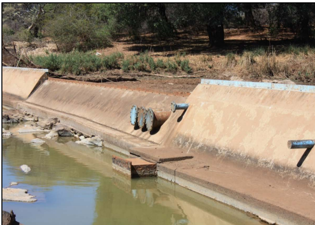
Figure 5.4: Gauging weir A6H035 in the Mogalakwena River
