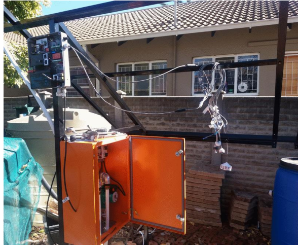
Figure 3.19: Monitoring and control system, and electrical panel during installation.
