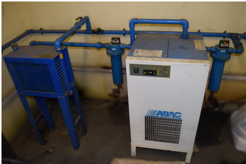
Figure 64: After-cooler unit (left) and air dryer unit (right)
