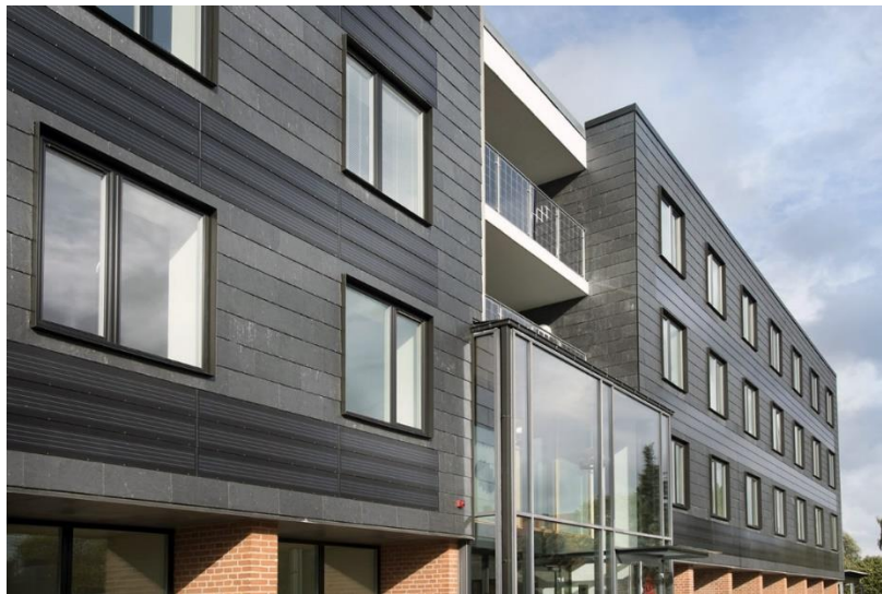
Figure 2.4: PVs installed as façade: BIPV type (Metsolar, 2022)
