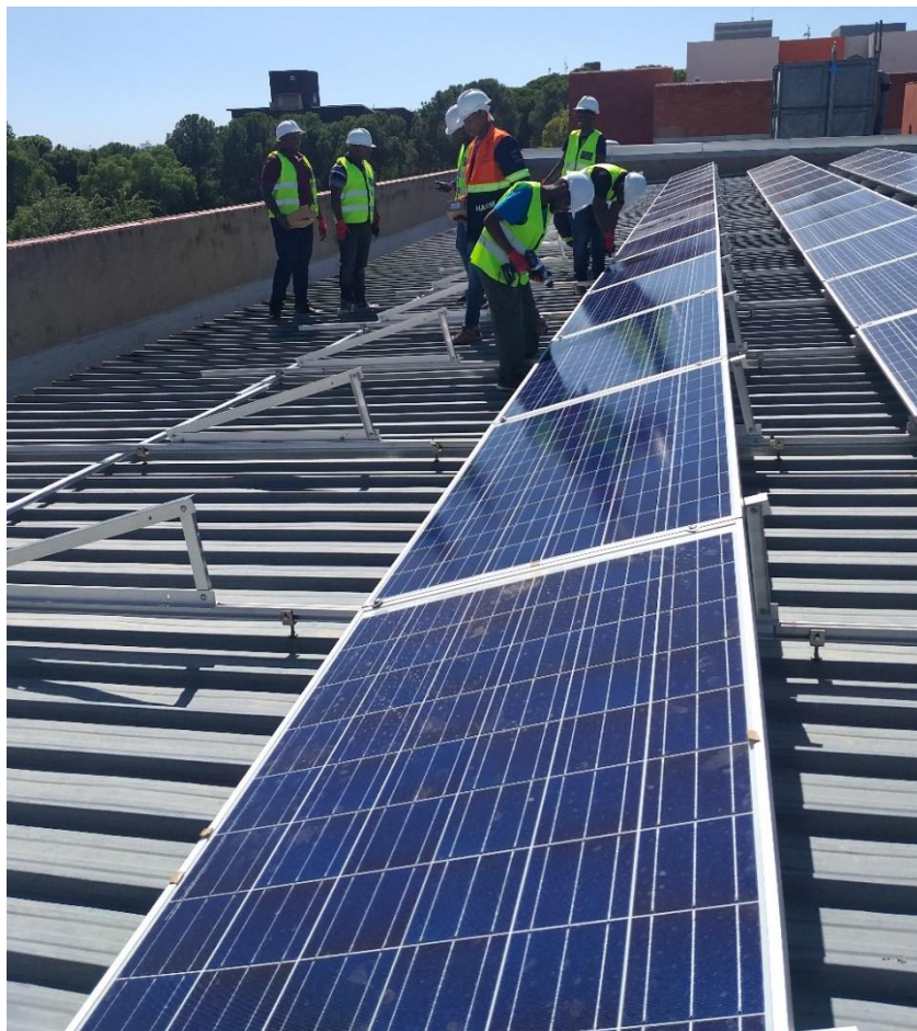
Figure 5.5: PVs installed by students at CUT
