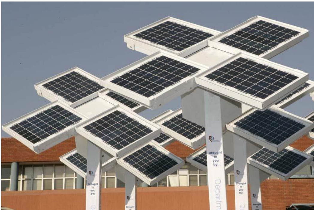
Figure 5.7: PV installation called 'Solar flowers' at CUT
