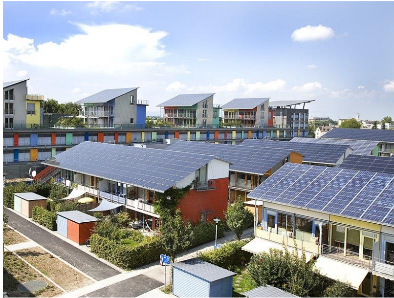
Figure 2.5: PVs installed as roof: BIPV type
