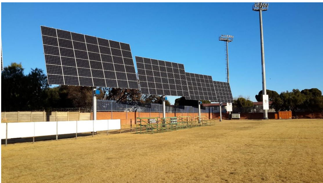
Figure 5.3: PV trackers installed on the sides of the football field at Bloemfontein Campus
