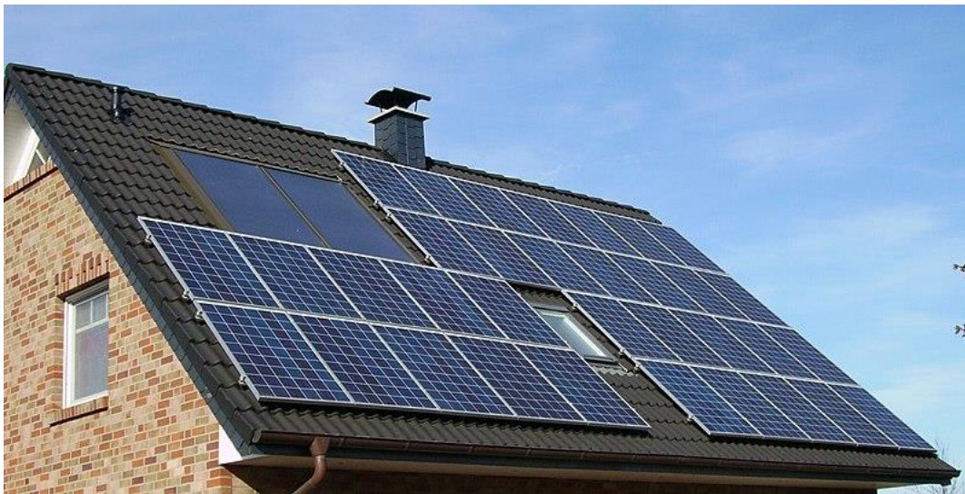
Figure 2.6: PVs installed on pitched roof: BAPV type
