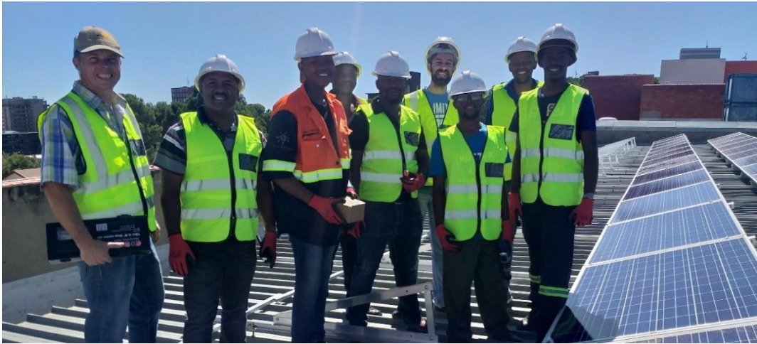
Figure 5.6: PVs installed by students at CUT
